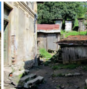
Acces deteriorat Damaged acces
