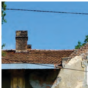
Acoperiș degradat Damaged roof
