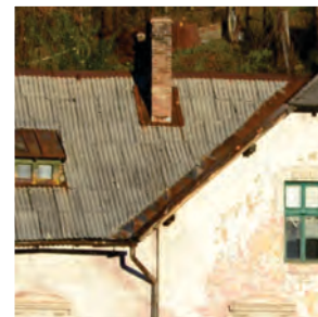
Acoperiș degradat Damaged roof
