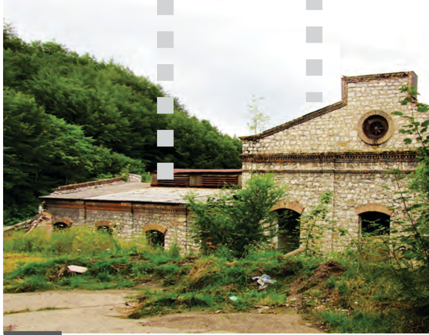
centrala termică puț I / thermal power station Pit no. 1
