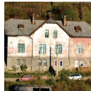
Fațade degradate Damaged fronts
