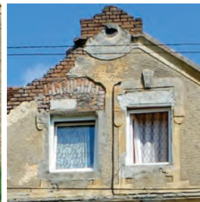
Detalii degradate Damaged front decorations
