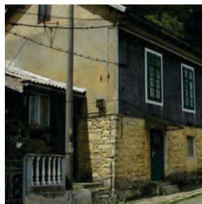
Acces deteriorat Deteriorated acces
