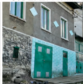
Detalii degradate Damaged front decorations
